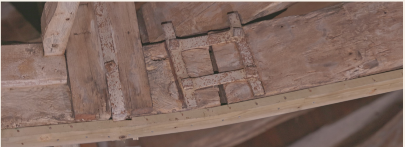
Iron strap connection at a principal rafter node. Mechanically fastened throughout. FennecMedia. CC BY 4.0.
